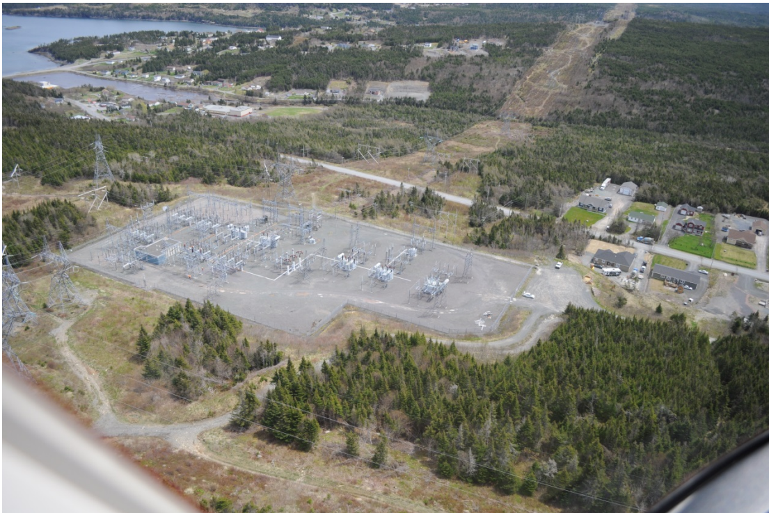
Western Avalon Terminal Station
